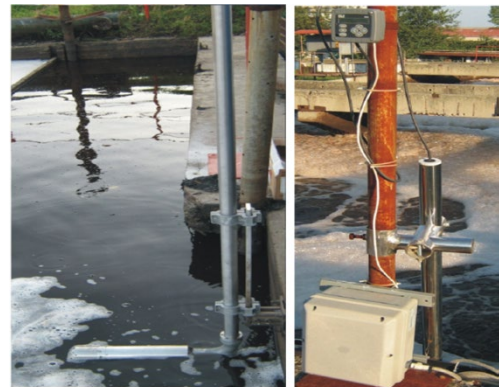
Control of the dissolved oxygen concentration in a wastewater treatment plant
